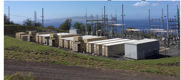
Standard containerized GSS ® grid storage solution
