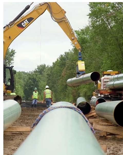
Construction of Consumer Energy's Saginaw Trail pipeline project in Michigan | Consumers Energy
