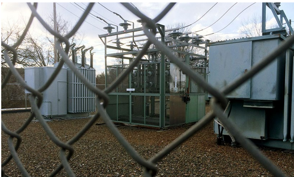
PECO substation near PJM headquarters | © RTO Insider LLC
