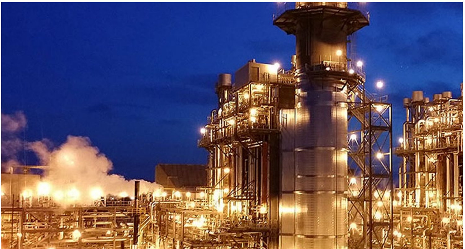
Panda Power Funds’ Sherman Power Project, one of three new gas plants it built. | Panda Power Funds
