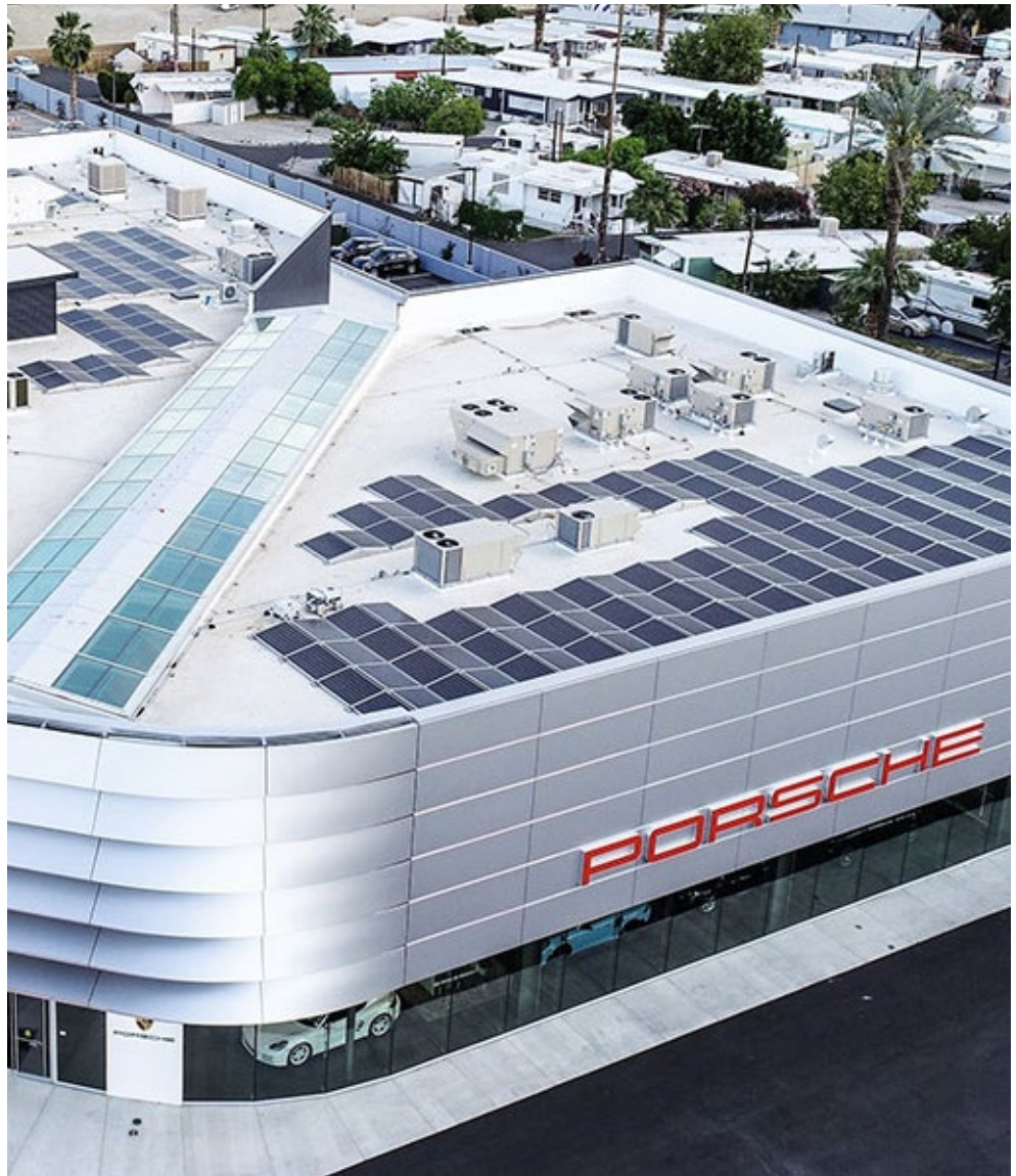
Many distributed energy resources, such as rooftop solar arrays atop commercial and industrial buildings, are too small to participate in wholesale markets directly and must be aggregated. | Renova Energy
