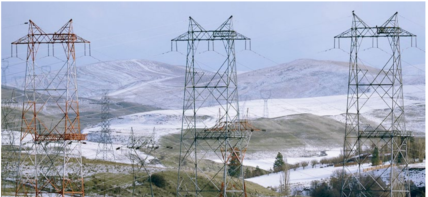
BPA transmission lines near The Dalles Dam. | © RTO Insider
