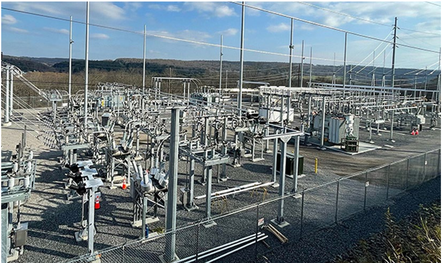
New York State Electric and Gas (NYSEG) in November 2021 completed its replacement of the Willet substation near Binghamton. | ISO-NE
