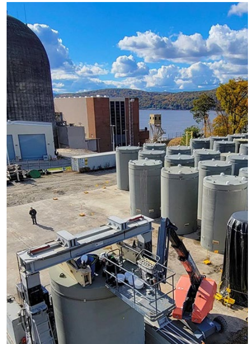
The exiting pad will hold 75 casks and a new expansion pad will hold an additional 52 casks. | Holtec
