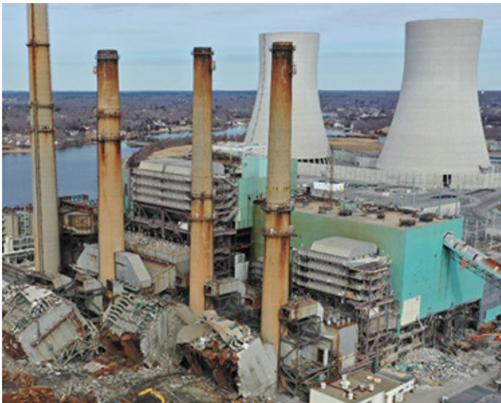
Brayton Point demolition underway in February 2019; implosion of the cooling towers is targeted for April 27. | Brayton Point Commerce Center
