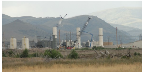
Dave Gates Generating Station | Corval Group
